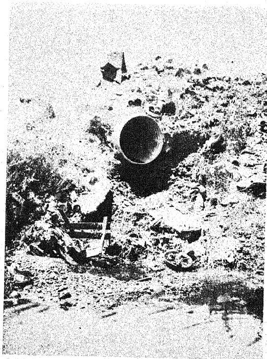
Figure 20. Upper end of a highway culvert placed too high for drainage. This results in mosquito breeding pools upstream from the culvert
